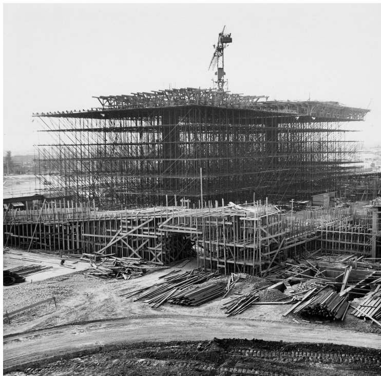
The National Sports Complex (Olympic Stadium), Phnom Penh under construction, 1963. Collection Vann Molyvann
